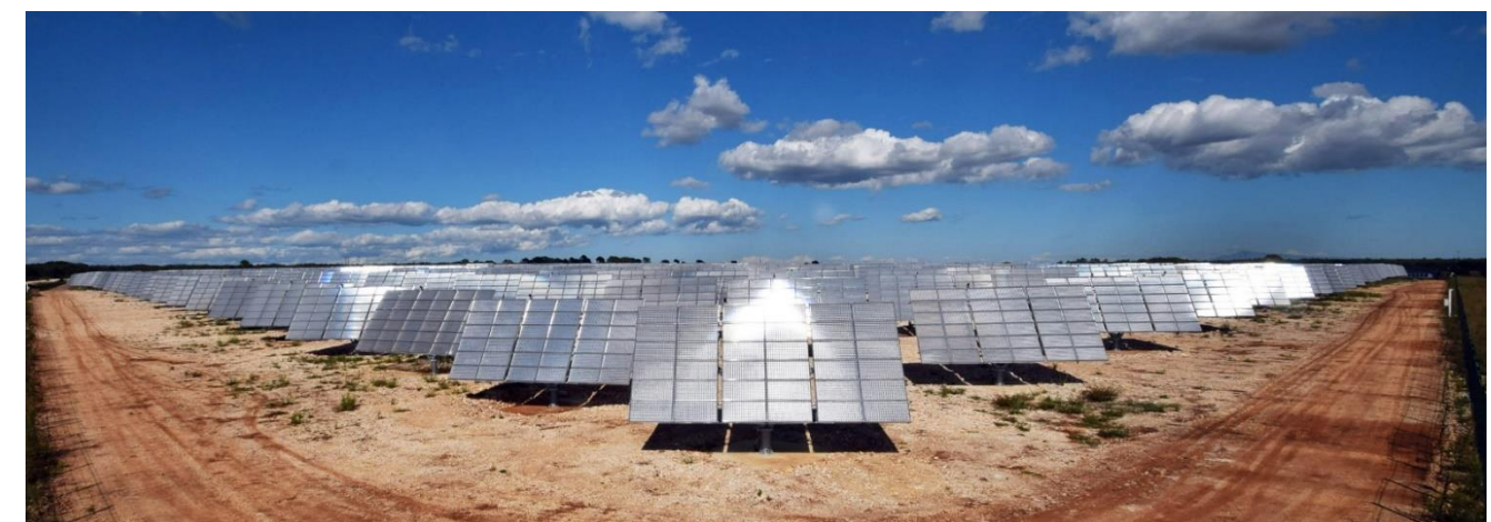
Figure 13 : Centrale photovoltaïque URBASOLAR (source : URBASOLAR, 2022)
